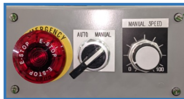
LOCAL CONTROL PANEL
